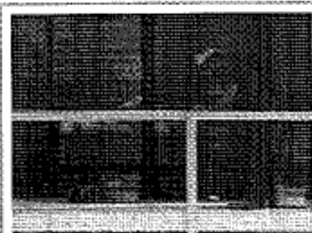
A construction worker is seen repairing damage to the apartment at 2 Secord Avenue on Friday, August 29.
