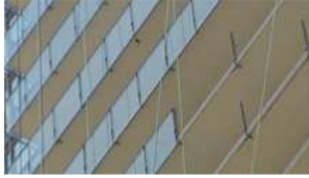
A screen shot of some of the balconies under repair at the Murano condominium complex on Grosvenor Street in Toronto, where several panes of glass have fallen from the structure.
